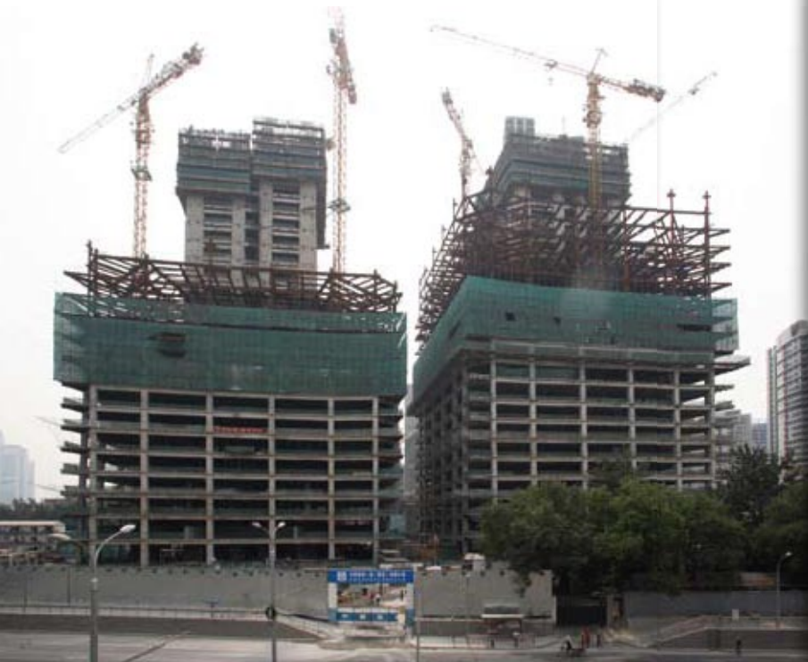
Self climbing formwork for central core walls and structural steel erection for floor plates
