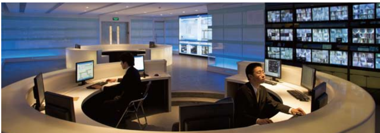
Building Management System (BMS) central control room for operation and monitoring of building services and security systems
